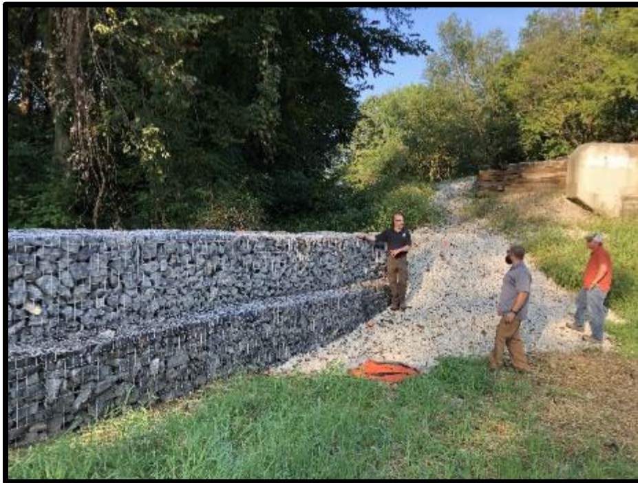
Photo of the Gabion Basket Barrier at the Ohio & Erie Canal. Source: OH DNR
