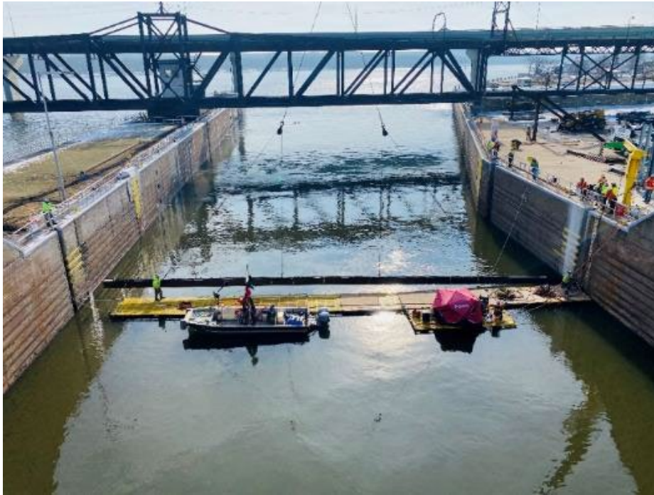
Figure 17 — Soundbar Installation – Lock No. 19 (Keokuk, Iowa)
