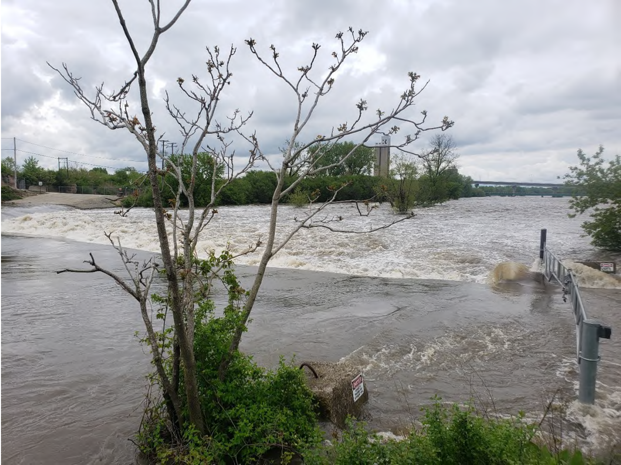
Picture 2: Picture of water flowing over the low water crossing road on the way to the Cargill boat ramp. The picture was taken May 18 th , 2020 looking south-southeast. The flow over the road is unlikely to allow fish to move upstream given the conditions.
