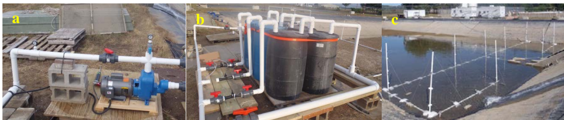
Fig 2: a) pump feeding water from the pond to the CO 2 infusion system, b) the CO 2 infusion system, and c) the discharge manifold.
