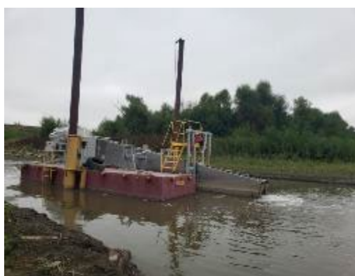
Figure 40 — Mobile Steeppass Fish Ladder with Scanner
