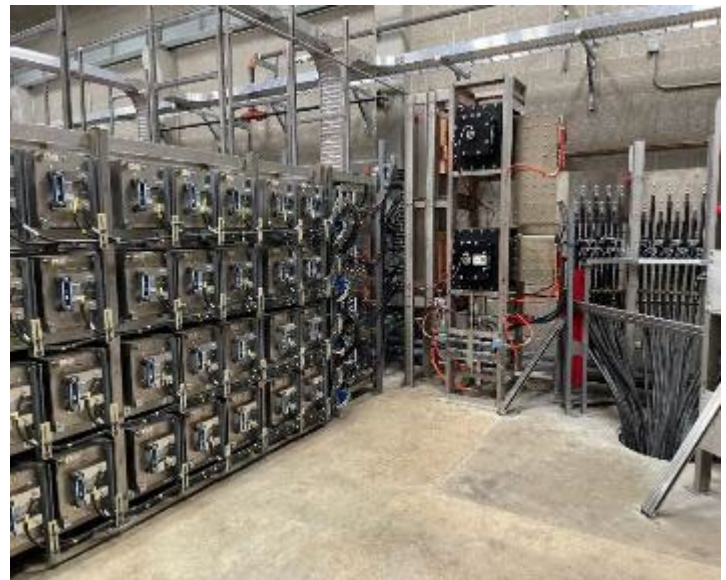
Figure 3 — Bank of Capacitors
