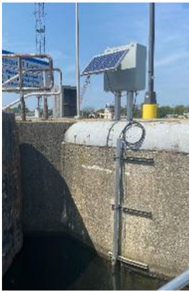
Figure 29 — Real-time Telemetry Receiver
