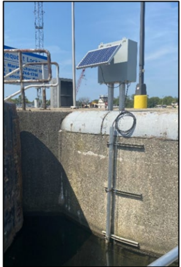
Figure 31 — Real-time Telemetry Receiver
