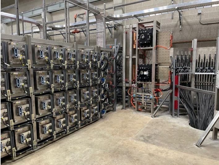
Figure 2 — Bank of Capacitors
